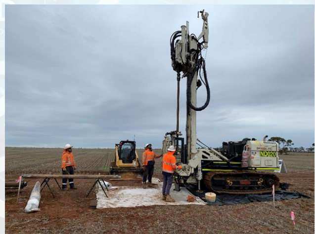
A sonic drill rig in action. This technique utilises ultrasonic vibrations with slow rotation to cut through the ground to obtain a 7-inch diameter core which is a larger sample suitable for metallurgical test work.
